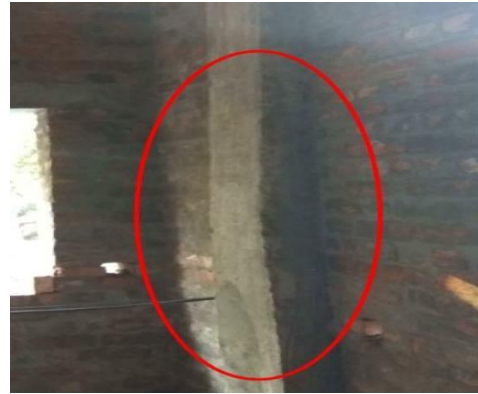
Figure 8. Non-verticality of column
