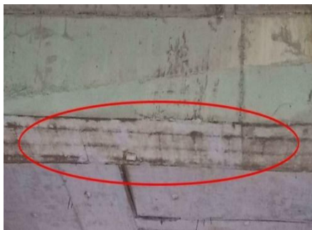
Figure 5. Reinforcements exposed in beam
