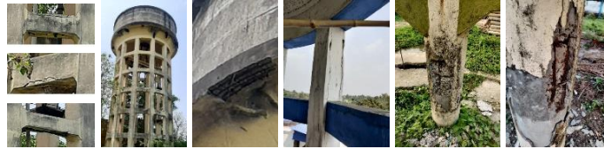
Figure 1. Typical RCC OHRs and their various Distressed Structural Elements subjected to Corrosion
