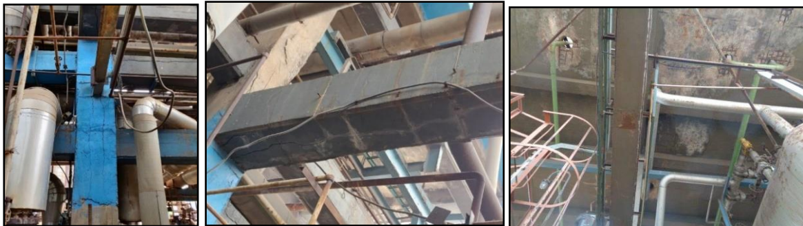
Figure 7. Deteriorated Structural Column, beam & slab before repair
