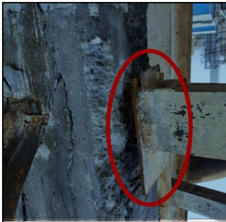
Figure 3: Steel beam came out along with inserts
