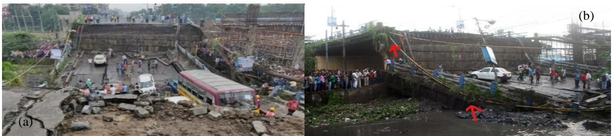
Figure 3. (a) Collapsed Girder; (b) Wild overgrowth of Majerhat bridge
