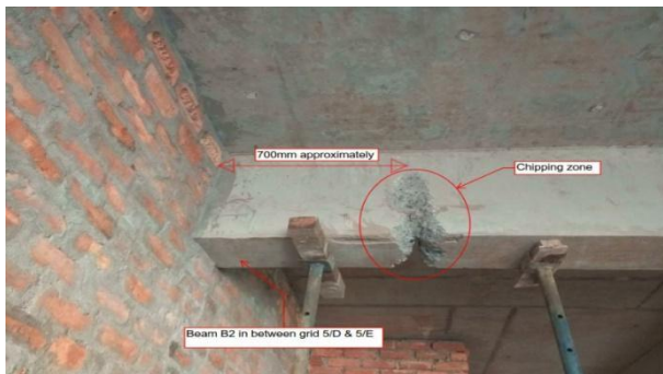
Figure 12. Chipping of Concrete at Beam Marked B2
