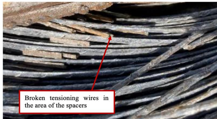
Figure 6. Tensioning wire bundle with wire breaks in the area of the spacers
