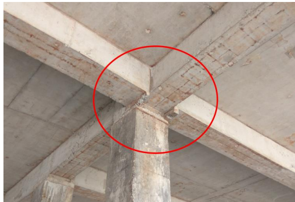
Figure 4. Beams are eccentric at the beam-column junction
