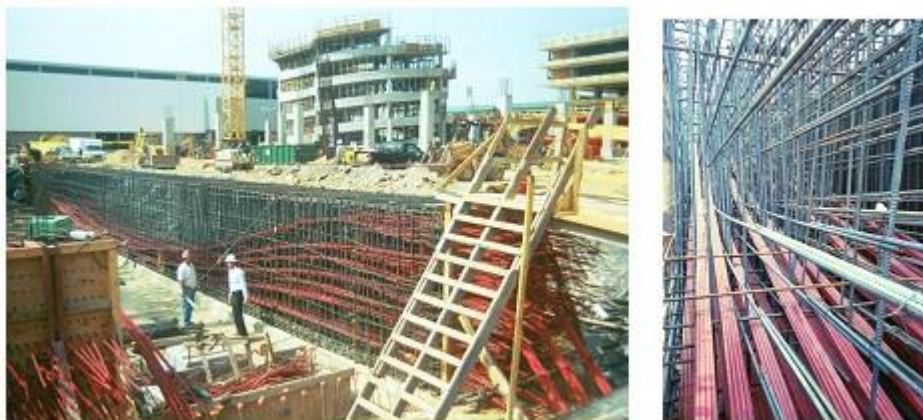
Figure 5. Transfer Girders that bridge over ITT Tunnel at Bush IAH Airport (Courtesy – Suncoast Post-tension Ltd)
