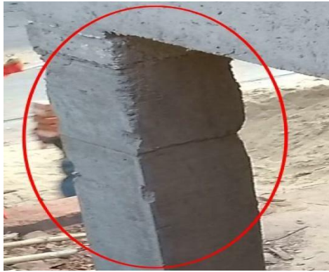
Figure 7. Non-verticality of column
