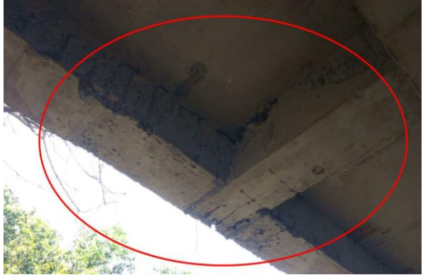
Figure 3. Reinforcements exposed in beam
