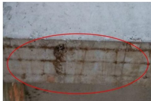
Figure 6. Reinforcements exposed in beam
