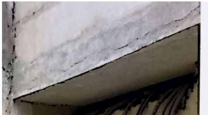
Figure 3. Cracks induced by reinforcement corrosion
