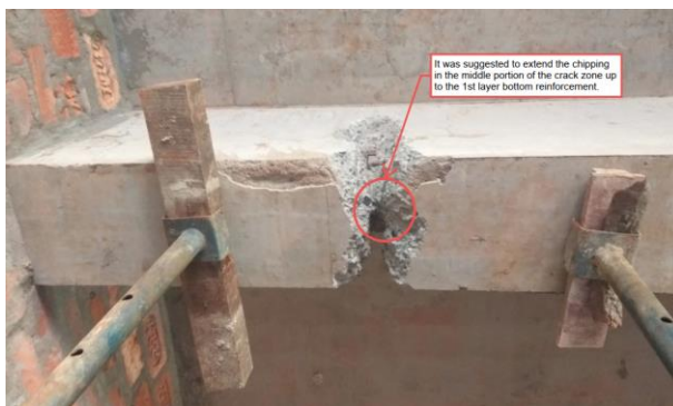
Figure 14. Chipping of Concrete at Beam Marked B2
