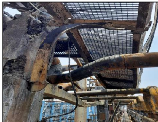
Figure 6. Steel bracket twisted and lost its connection
