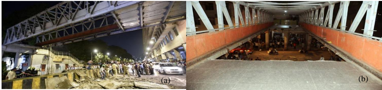
Figure 2. The CSMT bridge failure of the secondary beam [Subramanian and Abhyankar (2019)]
