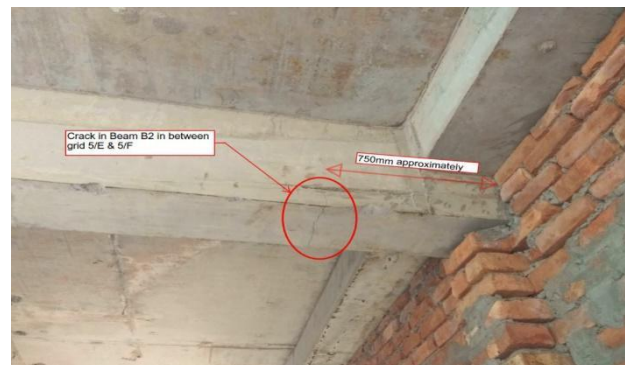
Figure 15. Crack in Beam B2
