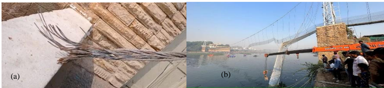
Figure 1. (a) The rusted steel cable; (b) Collapsed image of the bridge
