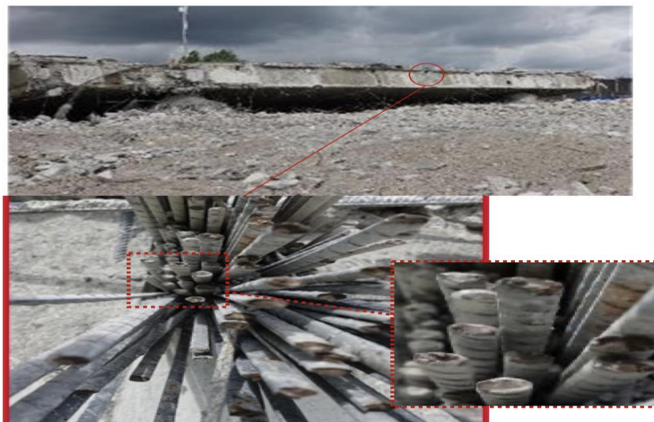
Figure 4. Tensioning wire bundle cracked due to hydrogen-induced stress corrosion cracking in beam 3 bay 2.2 near support C
