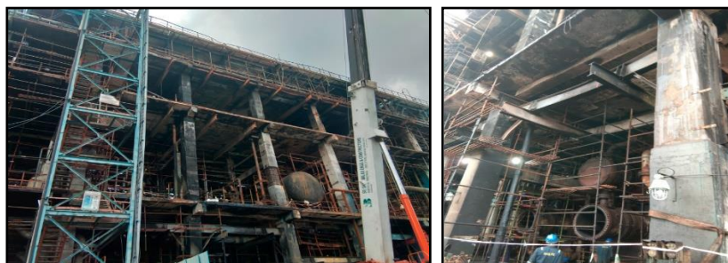
Figure 1. Images after the fire Incident
